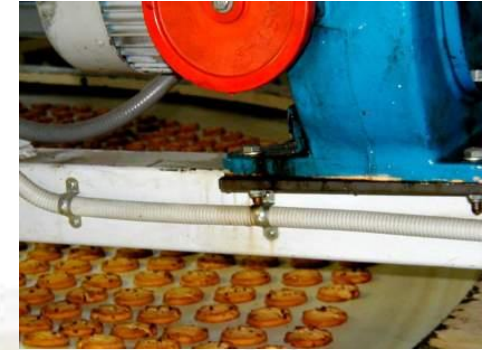
Leaking Gearbox above the food conveyor
