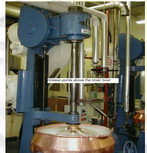
Grease bearings and grease points above foodstuff
