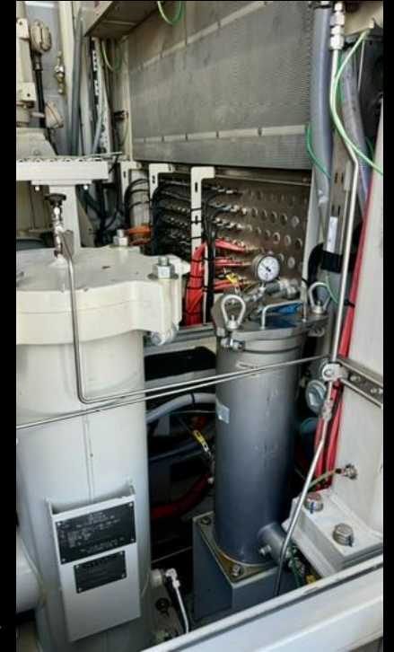
Resin Filtration installed inline on a gas turbine
